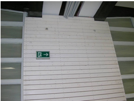
Figure 9: Cameras hidden behind cladding
