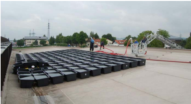
Figure 13: Artificial load on the roof of the school gym in Murnau, consisting of 154 buckets of the size of 90l, filled with water
