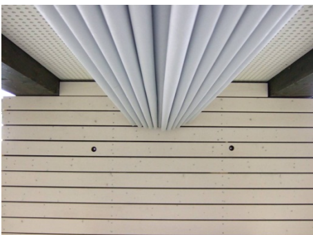
Figure 11: Reference points hidden behind cladding
